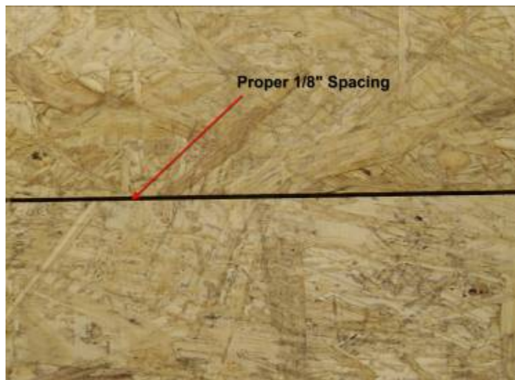
Correct installation of Advantech T&G Edge
